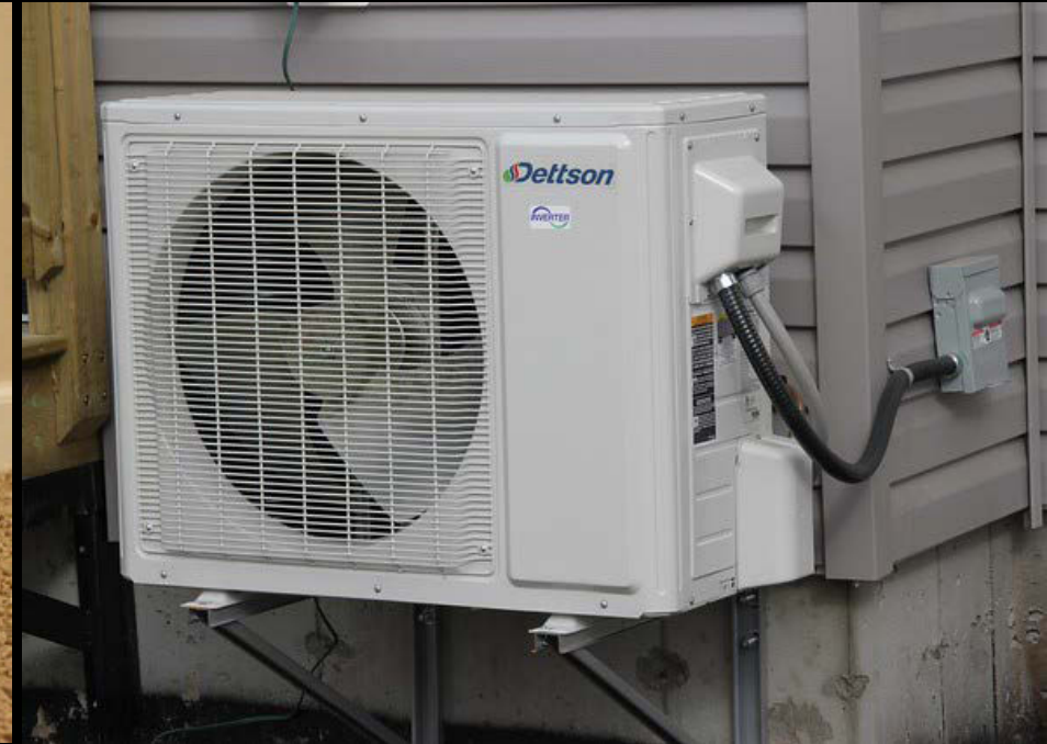
Air Source Heat Pump
